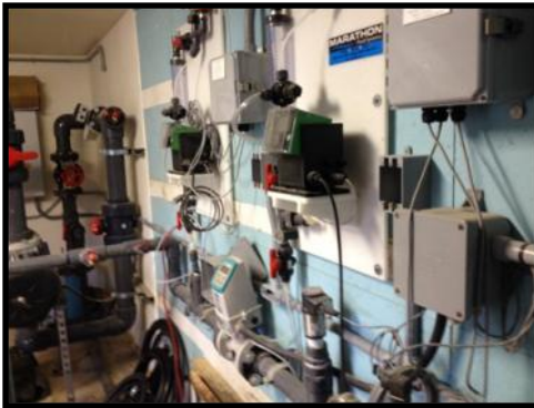
This Picture is Inside Division Road Well House; Process Related 2013
