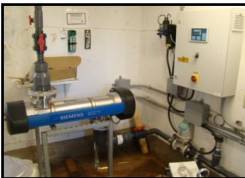
Water Treatment Ultra Violet System at Town Well on Beeches Road 2013
